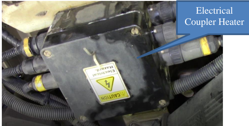
Figure 2.21, Electrical Heater, Courtesy of Metro Transit
