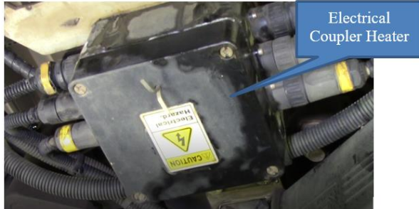
Figure 3.17 Coupler Heater, Courtesy of Metro Transit
